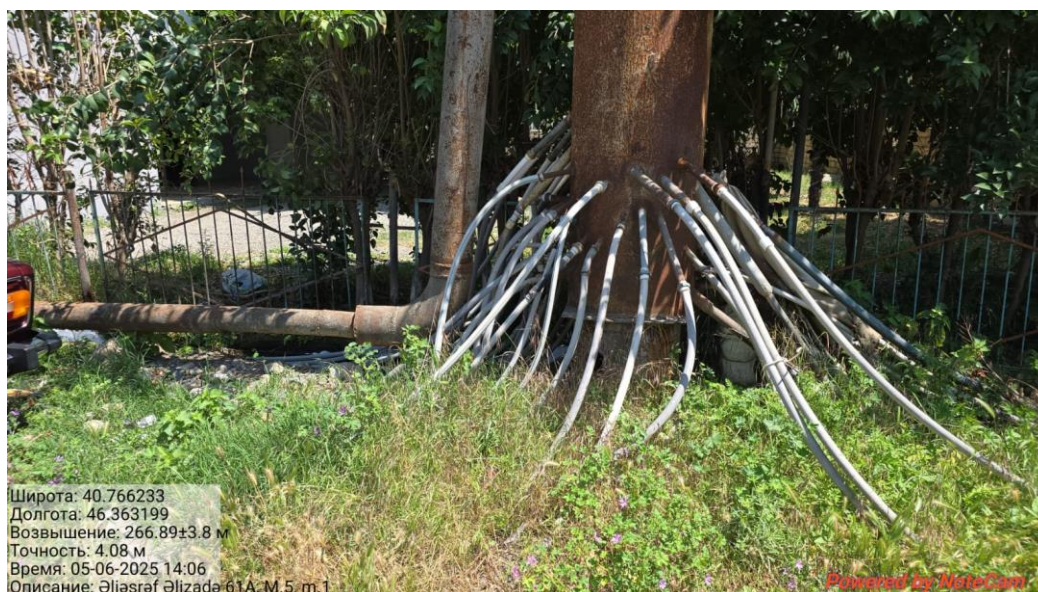
Figure 47. Water distribution infrastructure in Ziyadli village
